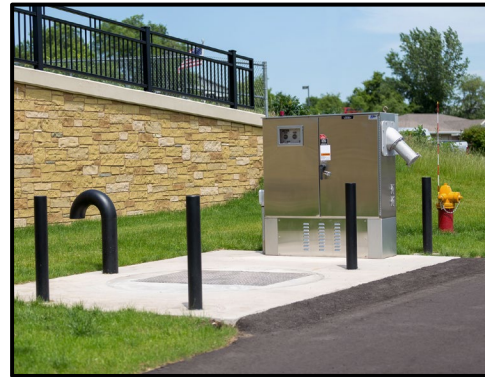
Sewer Lift Station
